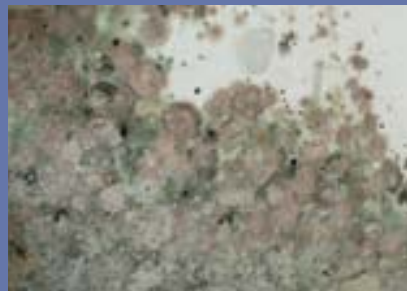
In order to remove areas of fungal growth it is recommended that experts are called in
