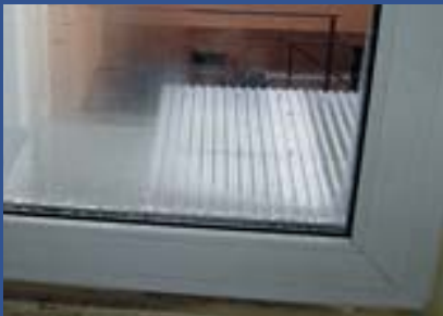
From water condensation to fungal contamination is a short step
